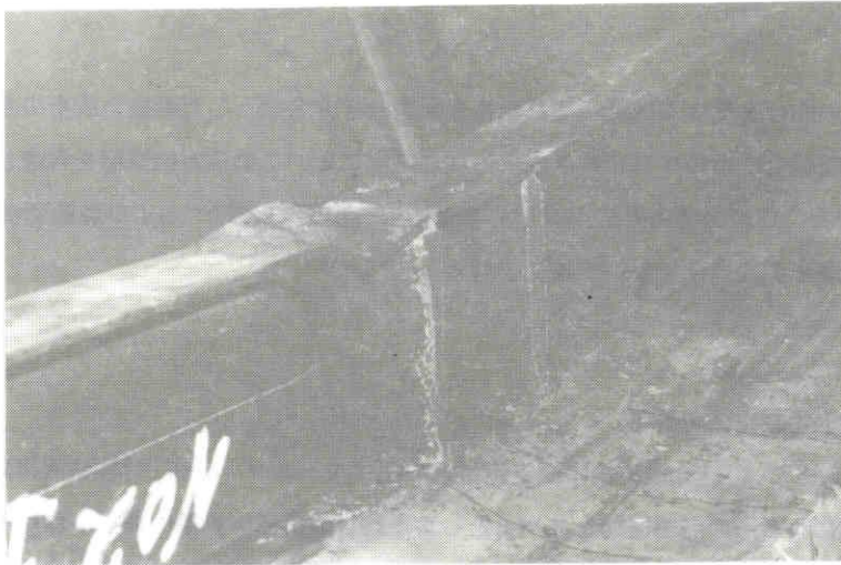
(a) Flange Local Buckling.
