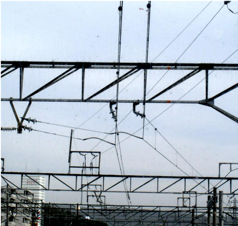
1-1; 電車の架線の切り替え(a relay of the electric string cables, @ JR-Kozoji Station.
