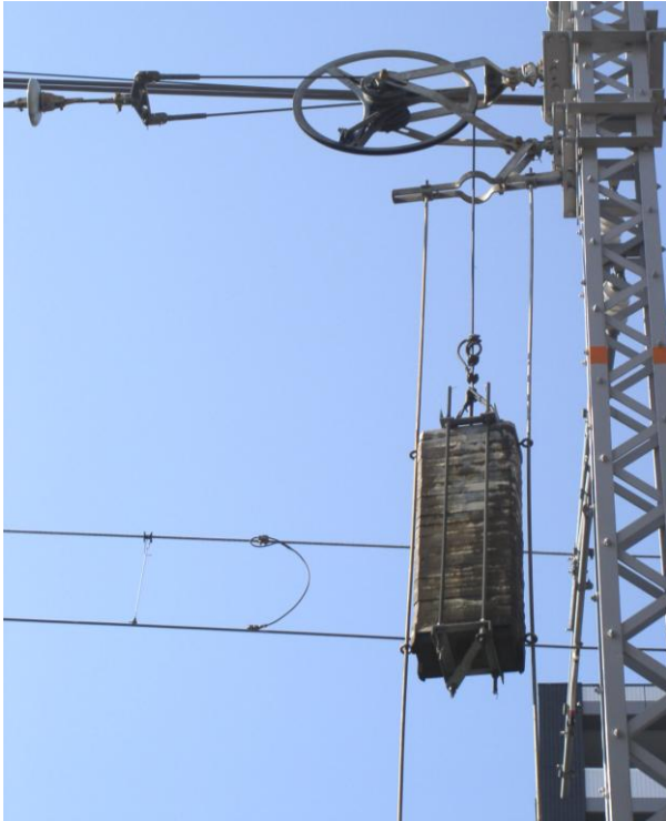
1-2(a); 電車の架線の張力は約 500kgW( Torque, Leverage) , @ JR-Ozone Station. An electric string placed under a tension of 500kgW.
