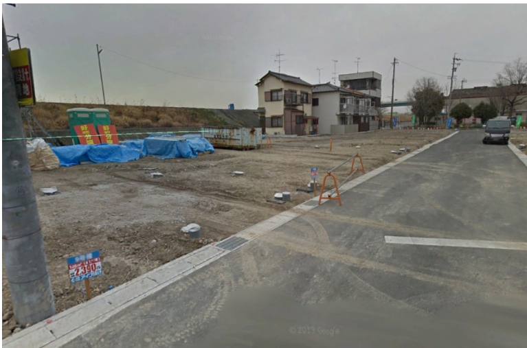
Figure 5-20 February 2012 construction on new housing complexes in Nishi ward near Shin River (google Earth street view photo)
