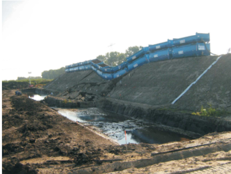
Photo 1. 1 The example of failure embankment over peat deposit (after Zwanenburg et al., 2012)
