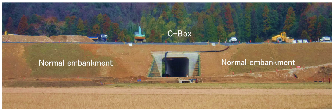
(b) Residual settlement considered (STA509, taken in 2013)
