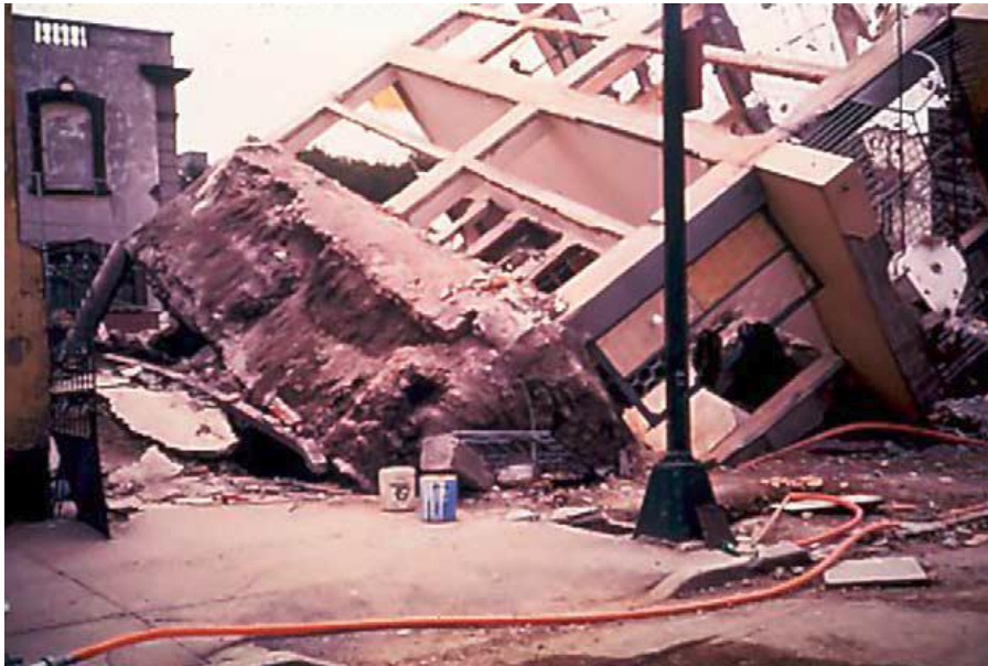
Fig. 4.1 Overturn damage of upper structures due to decreased bearing capacity of clayey foundation
