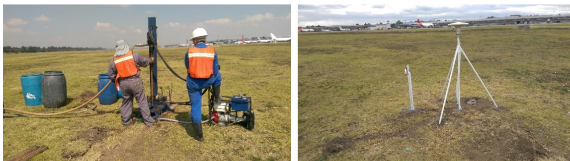
Figure 14. Deep-drilled braced monument (AEDO station).
