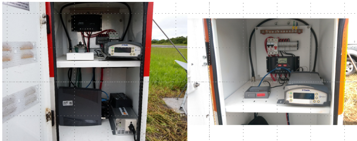
Figure 20. Instruments stored inside the enclosure. Left, internet satellite link; right, radio-modem
